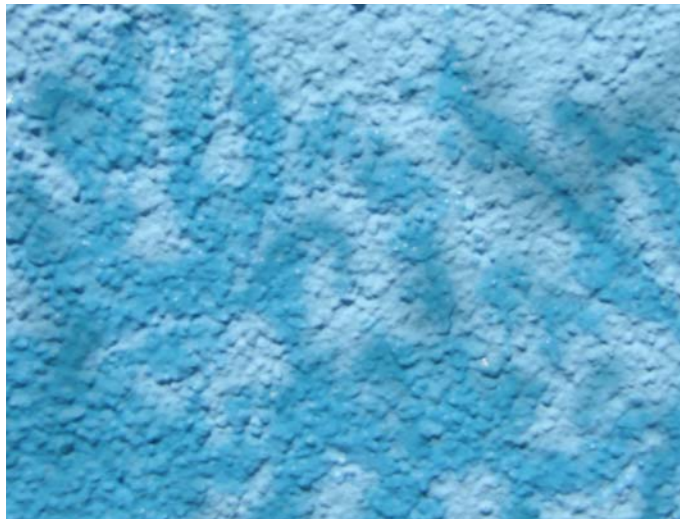
dirt gets into paint structure
