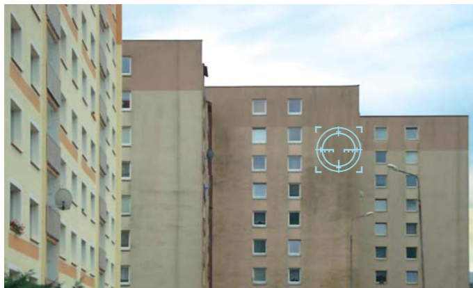
Unsecured plaster with biological contamination. Dirty and unaesthetic facade.
